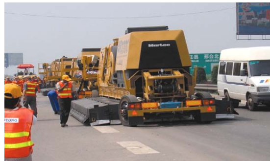
FIGURE 13 China – 2004 Heibei Province Shi-An Expressway Demonstration Project, 10 lane-km. Technology Transfer Completed to Chinese National Standards.
