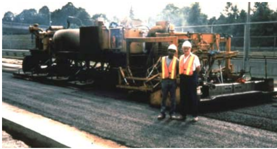
FIGURE 3 First Generation HIR Heater. Scarification of Old Asphalt Pavement Prior to Placing Overlay, Toronto, Early 1980s.
