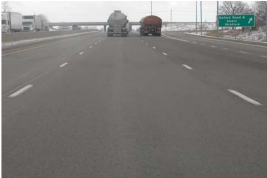
FIGURE 18 Martec AR2000 HIR Section, 2005. Very Good Ride Quality and Good Surface Condition.
