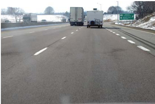
FIGURE 22 Mill and Fill with RHM Section, 2005. Very Good Ride Quality With Some Low Severity Deterioration.
