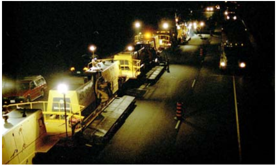
FIGURE 14 Martec AR2000 HIR Equipment (Figure 7) Working at Night With Traffic on the Ontario Highway 401 Demonstration Project, September 1999.
