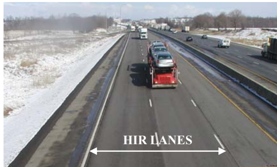
FIGURE 17 Current Condition of the Martec AR2000 HIR Section in February 2005 Showing the Excellent Condition of the Two Lanes Involved.
