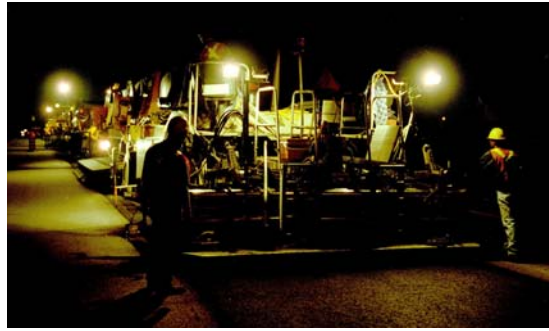
FIGURE 15 The Martec AR2000 HIR Section Involved Two Lanes (5.6 lane-km) With Processing Depth of 35 mm and Compacted Remixed Premium Mix Depth of 50 mm (8).
